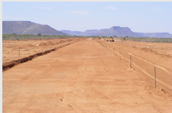
► Progress with new landing strip. Photo credit: Dawie Fourie, SKA SA Karoo site manager, 21 April 2012.
